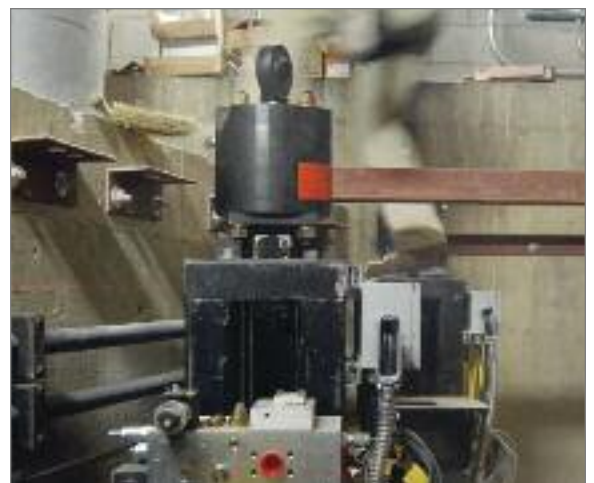
Theater stage lift
