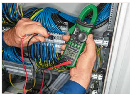
Current measurement in a control cabinet
