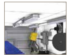
Full Electrical Service
