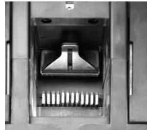
Magnum DS Breaker Contacts (Arc Chutes Removed)
